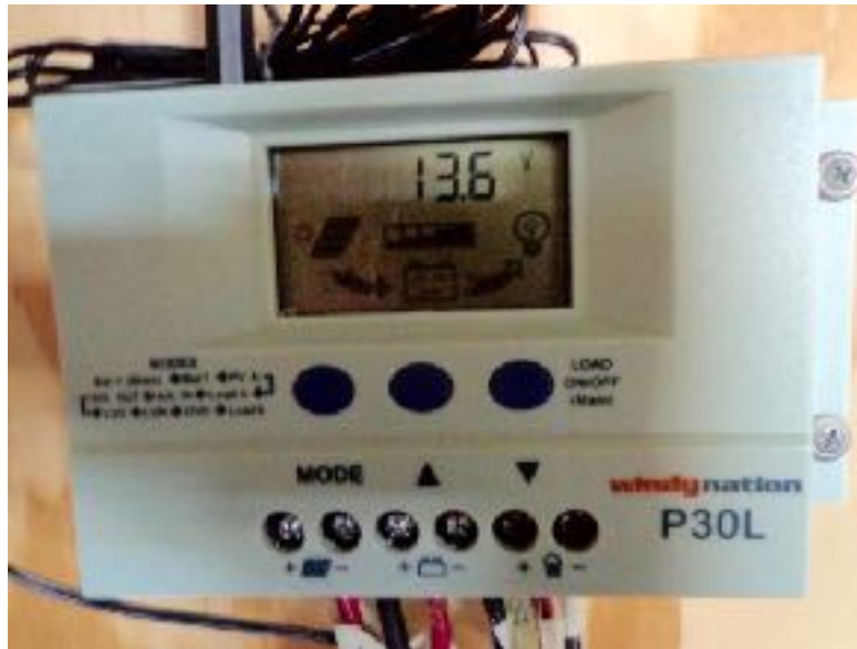
Controller shows Battery Voltage
