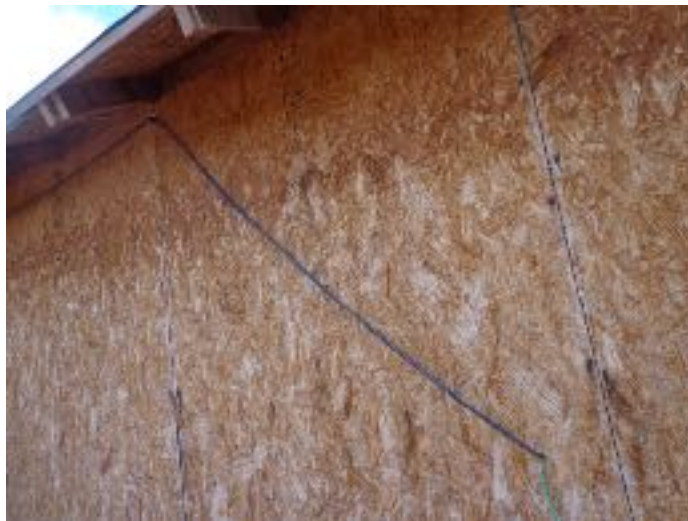
Wire into house
